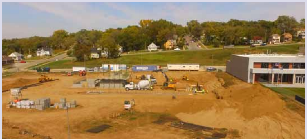
Construction is underway to build the new Academic Classrooms of Heelan High School.
